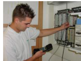
Stephen checks the telephone system
